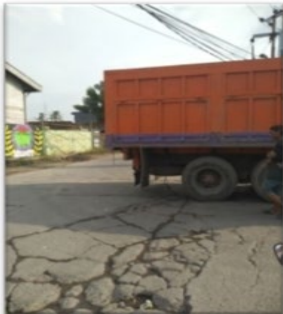
Picture 3. Condition of the Legok Street
